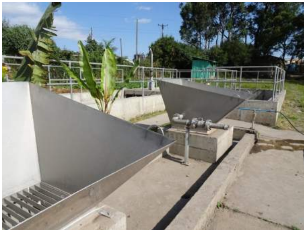
Figure 16 Reception area septage at Kality WWTP (Source: field visit WWX 1 November 2021)
