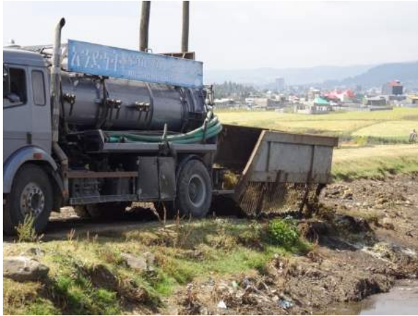
Figure 31 Erosion of banks of sewage ponds (Source: WWX, 2021)
