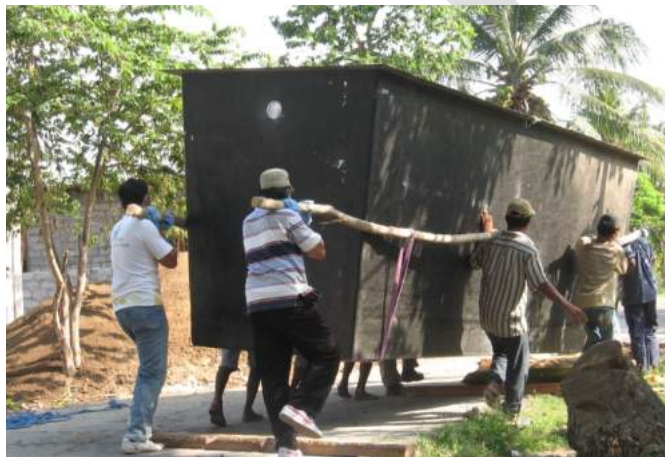
Figure 10 Transfer prefab ABR (Source: BORDA, 2012)
